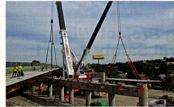
TAKING A DETOUR Traffic on I-93, which carries about 200,000 vehicles a day, was rerouted to alternate lanes during the bridge switch-outs.
