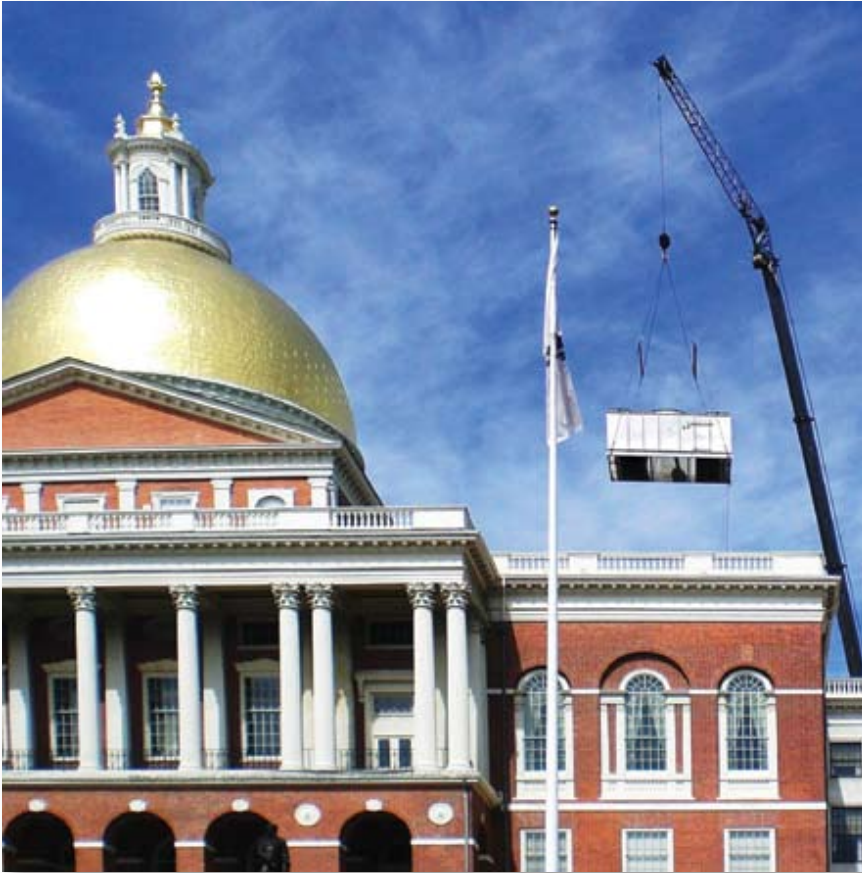
J.F. White's Mechanical Group replaced existing boiler and chiller tower with two 393 kbtu/h boilers and installation of 750-ton centrifugal chiller without disrupting activities at State House
